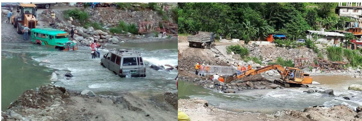
Figure 8. Along Halseman highway Sabangan to Sagada, (access point 1 from figure 1), after the bridge was washed out by river water due to typhoon Haima in 2016 (Source: Google.com)
