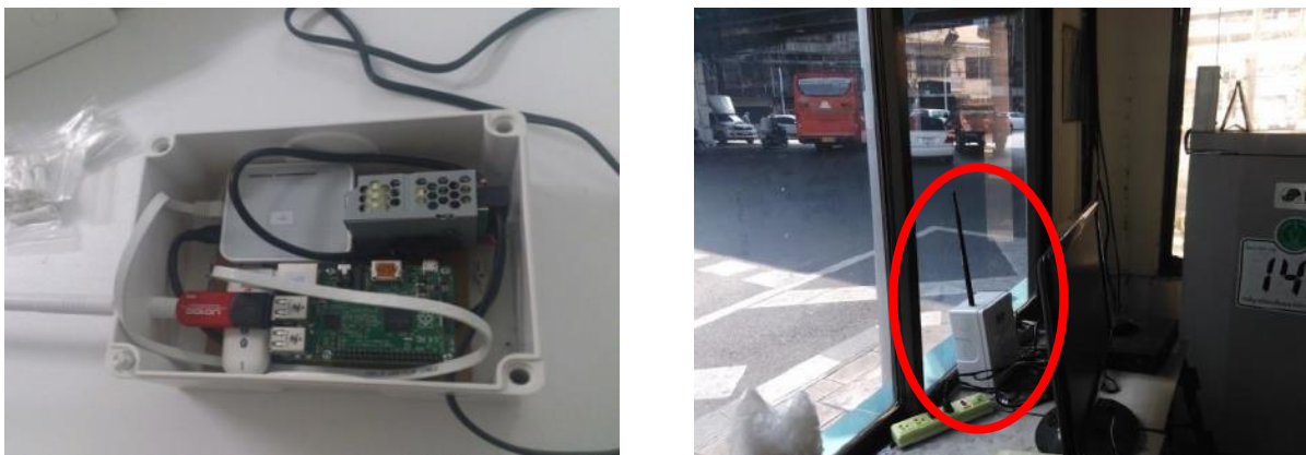
Figure 1. Bluetooth MAC scanner and installation place
